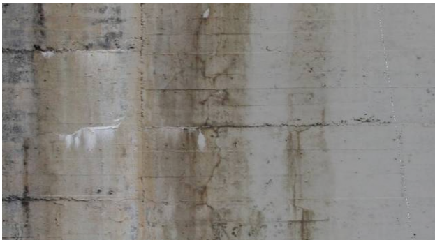
Figure 3. Picture of a defect captured with SCANSITES®
